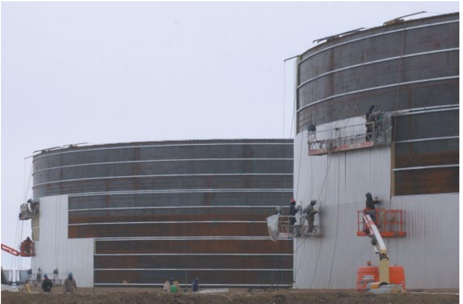
Fuller Austin: Storage tank insulation
